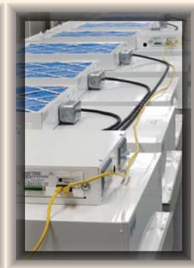
Fig. 3: SAMlink Control Housing Mounted on Master SAM Unit
